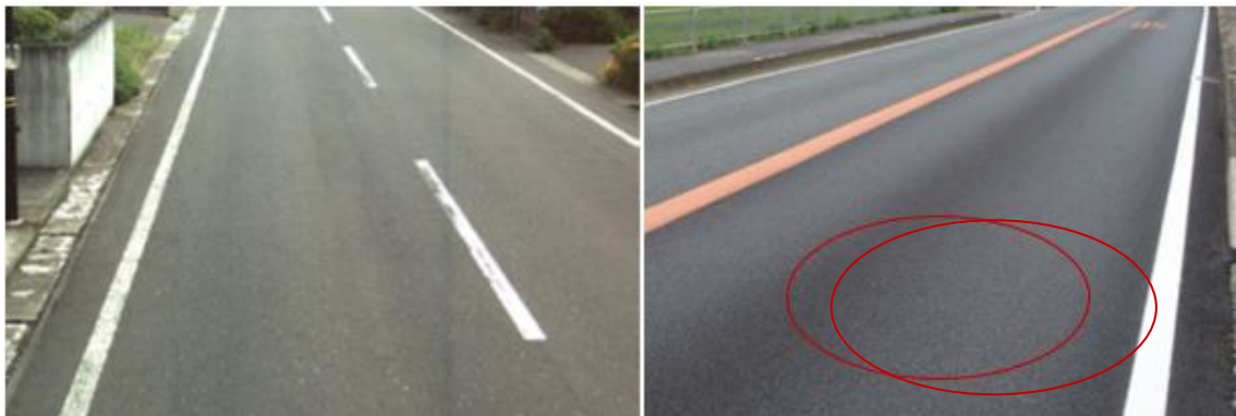
Figure 2: Correlation between road surface conditions and IRI (IRI=0 ~ 3): A condition of satisfactory asphalt paved road surface
