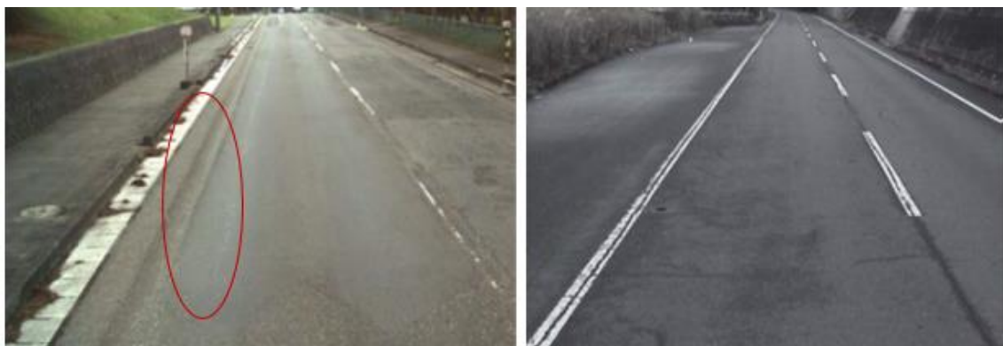
Figure 3: Correlation between road surface conditions and IRI (IRI=6 ~ 8): A condition that the paved road surface has gradually been eroded from bad to worse.
