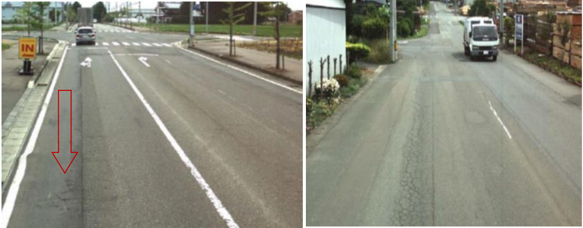
Figure 4: Correlation between road surface conditions and IRI (IRI=11 ~ 12): A condition that the paved road has already been eroded and it has resulted in a series of potholes.
